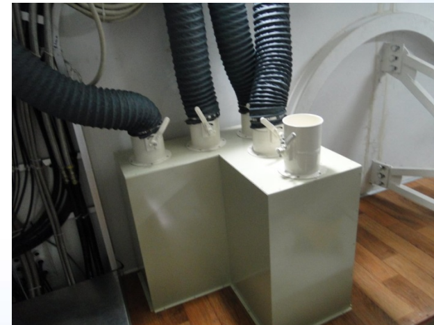
Distribution box for air ducts
