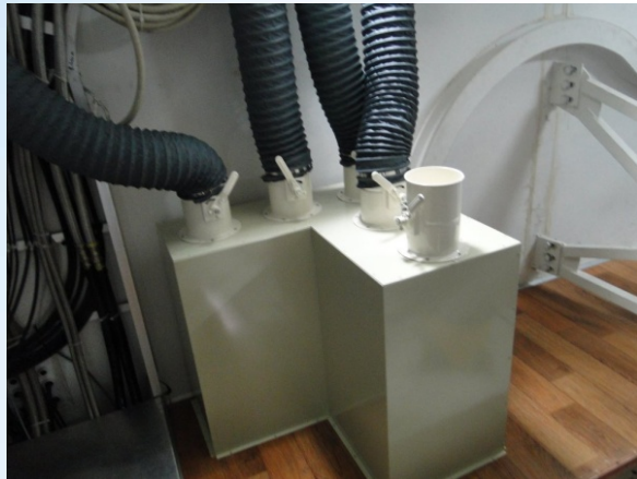
Air distribution box in RR for air discharge
