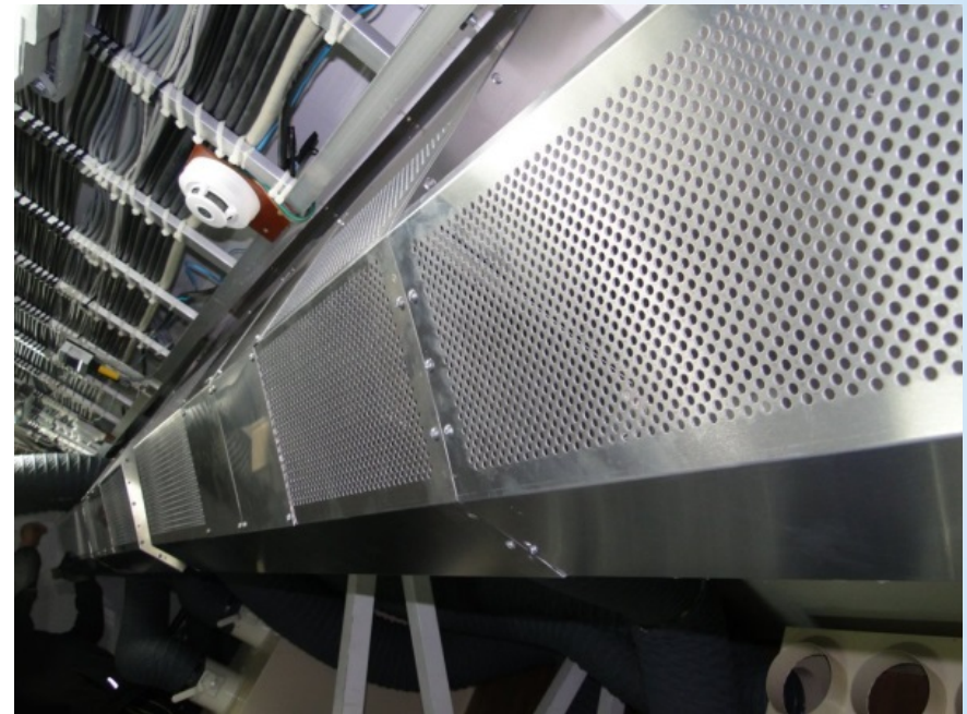
Perforated air ducts for air circulation
