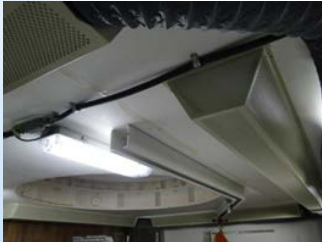
Perforated air duct in receiver cabin
