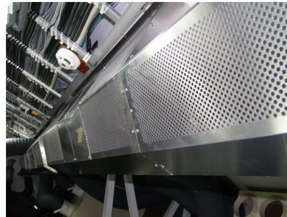
Perforated air ducts for air circulation
