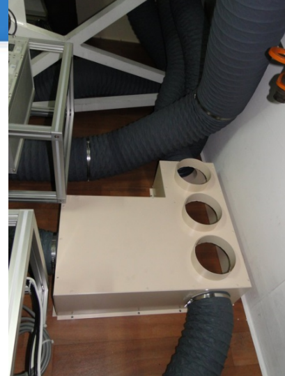
Inlet box for even air suction in receiver cabin
