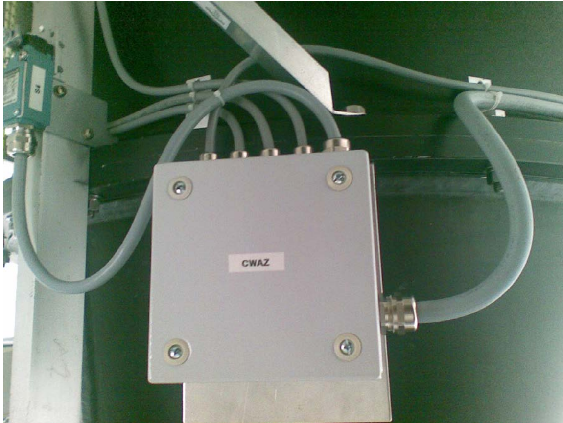
Azimuth limit switches distribution box
