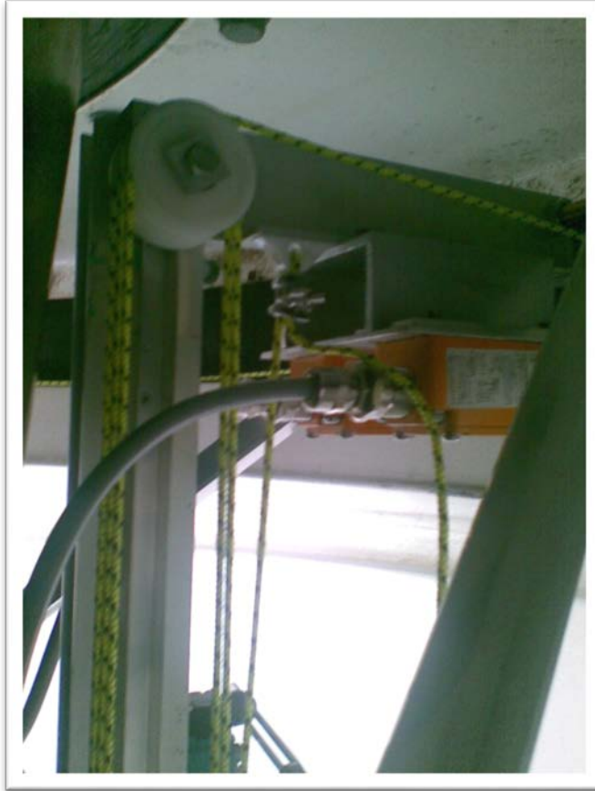
Azimuth hard stop switch assembly
