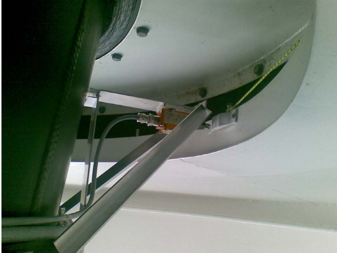
Azimuth CW limit switch, striker plate & hard stop rope October 2012
