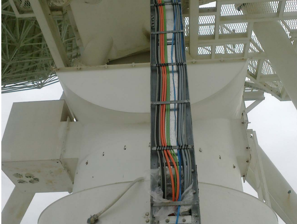
Elevation motor, stow-pin, position encoder & limit switch cables July 2013
